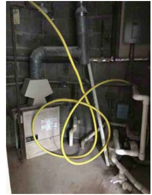
pool equipments room
