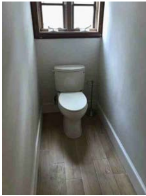
full bath# 3 -toilet
